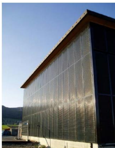
Fig 4: Unglazed flat plate collectors integrated on the façade (Energie Solaire)
